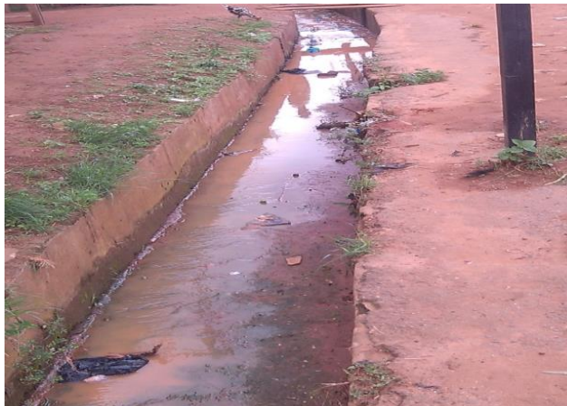
Figure 6: Open Drainage where feces are dropped
